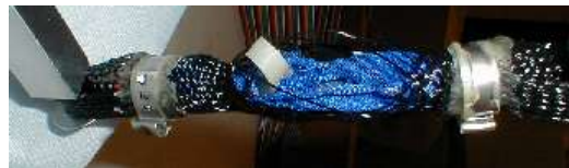
Figure 4: Catastrophic mesh integrity failure
